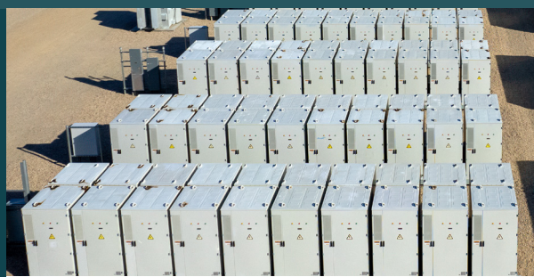
Example of a BESS. Final design will be confirmed through the development approval process.
