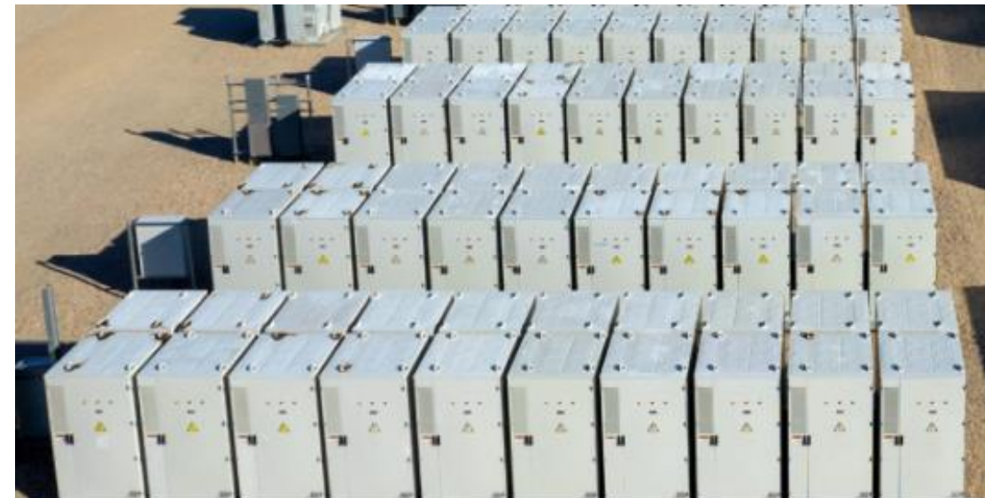
Example of a BESS. Design is not yet confirmed.
